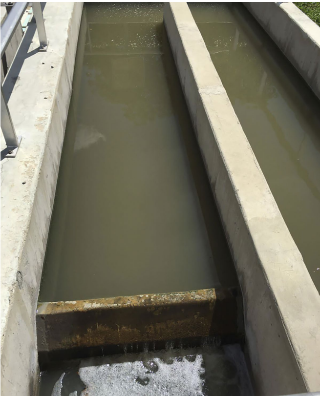
Appendix 5: Chlorination Chamber
